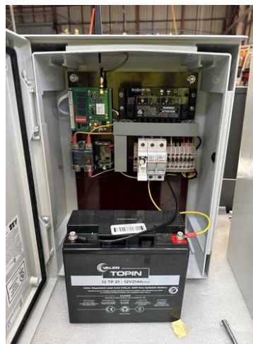
Sign Activated via Local Controller
