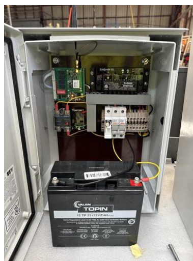
Sign Activated via Local Controller
